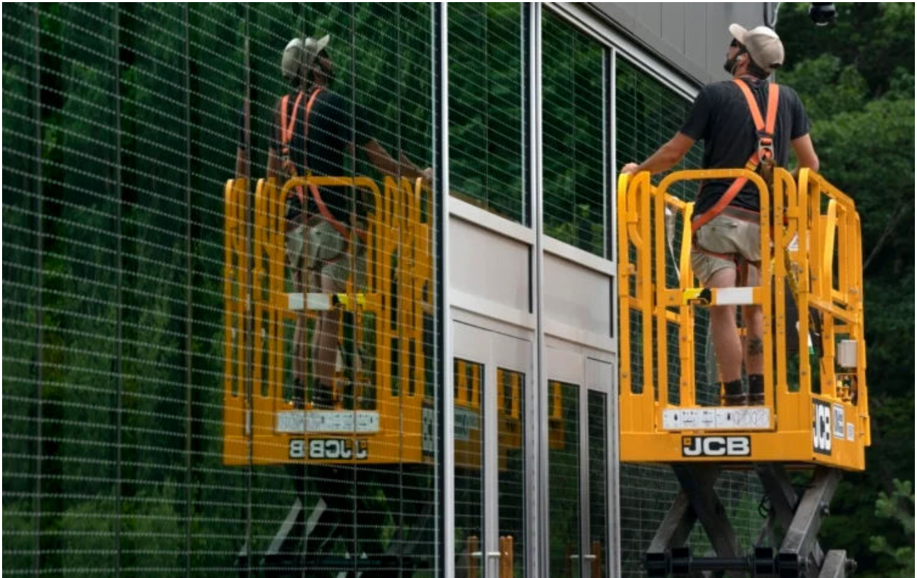
Cole Hutchison raises a lift to apply a laminate of dots on the windows of the new L.L. Bean headquarters in Freeport on Aug. 5. The dots help minimize bird collisions into the windows. Gregory Rec/Staff Photographer
