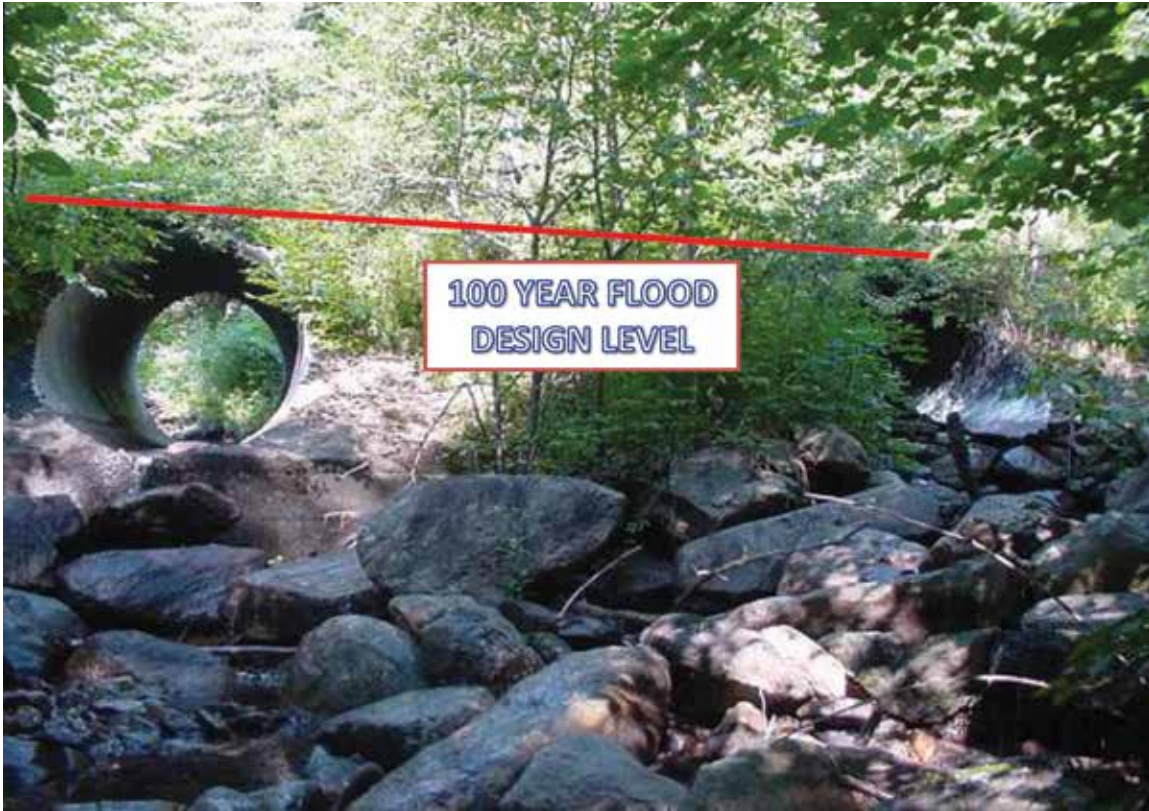
Figure 4. Typical hydraulic design double culvert over Jenny Coolidge Brook, May 2010. Green Mountain National Forest showing estimated height of 100-flood design discharge in red. Photo credit: Brian Austin, Green Mountain National Forest.
