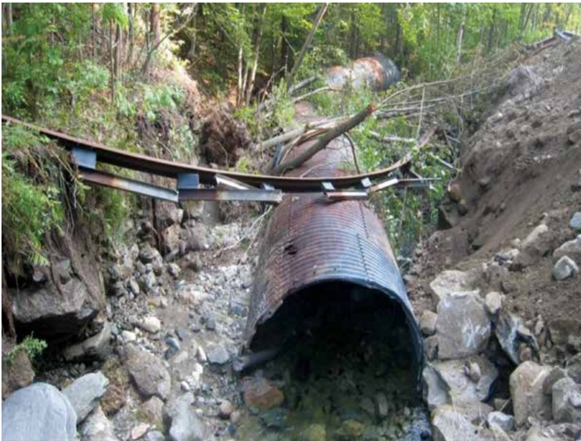
Figure 1. Road failure at a 3-m culvert placed within a 6-m bankfull width stream, Green Mountain National Forest. Photo credit: Dan McKinley, Green Mountain National Forest.
