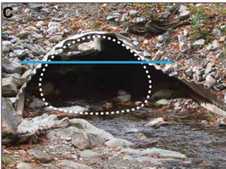
Figure 3. Sparks Brook road-stream crossing located on the Green Mountain National Forest, showing (a) original hydraulic design pipe-arch built in late 1960's, with a 2.5 m span and 1.9 m rise; (b) stream simulation design open-bottom arch structure built in 2010 with 4.5 m span, 1.62 m rise and footers extending 2.7 m below channel bed; (c) replacement structure after Irene flood. The blue line illustrates the actual peak flood water-surface elevation as well as the estimated peak flood elevation if the original culvert had been in place. Photo credit: Dan McKinley, Green Mountain National Forest.
